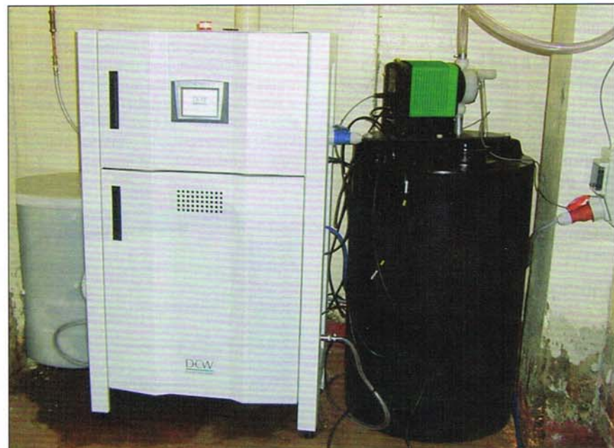
The DCW generator is located in the cold water boost room of the hospital's main boiler house.
