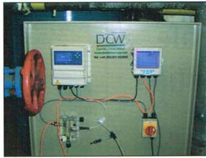
The standalone monitoring panel.
